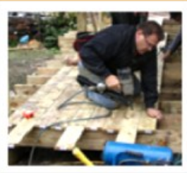
Neal, the general manager at Home Depot, works on constructing a new porch for the ministry house at our last workday
